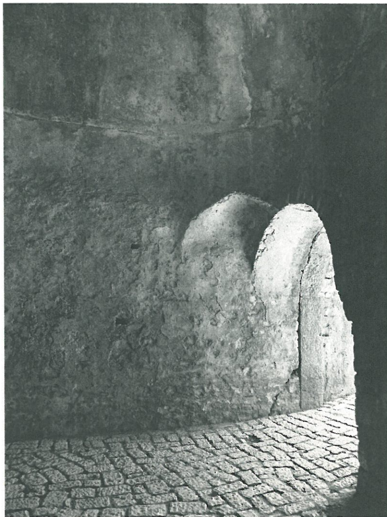
Fig. 2. Interior of Ottoman gate complex on eastern wall, with one of the dome squinches visible.
